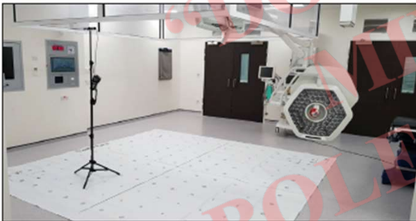
UCV canopy low level air velocity test
